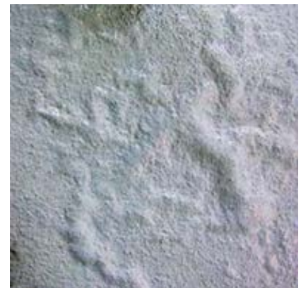
Figure 1: Traffic coating membrane blistering example
