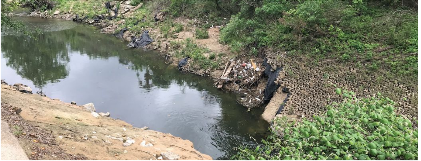
(Opposite) Buffalo Bayou experienced extreme erosion during and after Hurricane Harvey. (Top left) Long-duration high flows can undermine bridge abutments, such as this bridge at Saunders Road in Houston. (Top right) Structures can be undermined by sustained flows, as seen here on Spring Branch. (Bottom) High flows around an outside bend greatly affected existing erosion control measures on Spring Branch.
